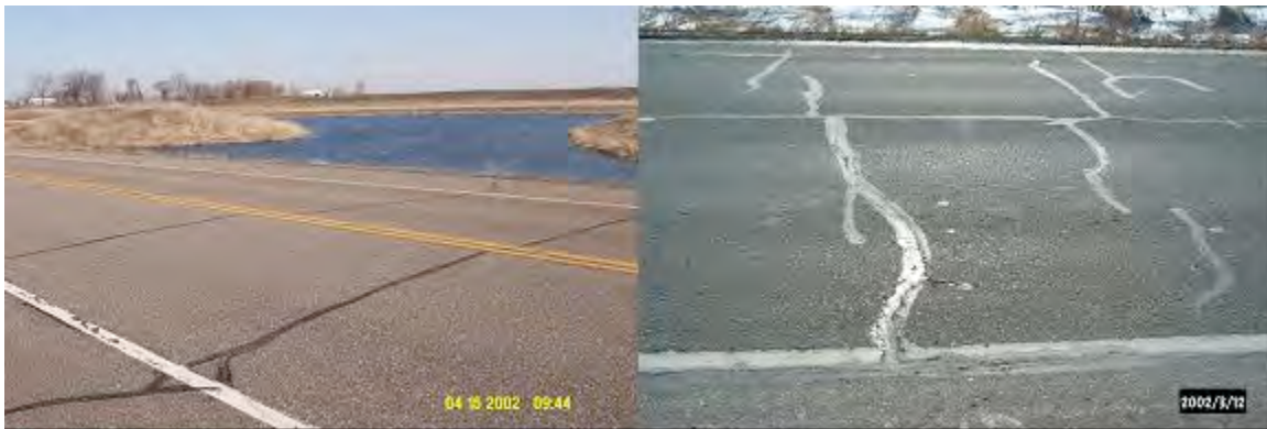
Figure 4. Typical Cracking Patterns on PG 58-28 (left) and 64-22 (right) Cells
