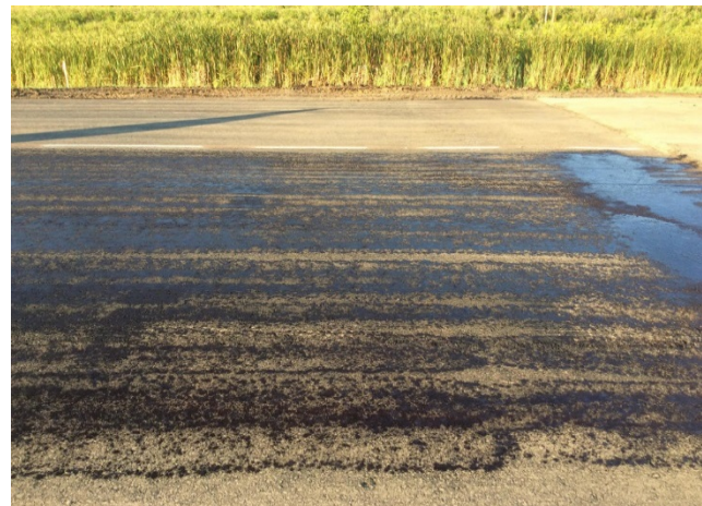
Figure 1.1-2 - Tack coat application at MnROAD 2016 construction – note this was not acceptable and was reapplied before paving.
